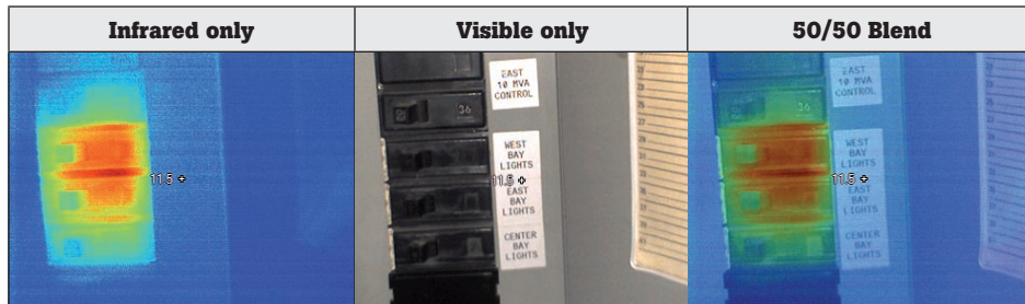
Figure 6. Equipment labels and the problem area can be read in an infrared and visible blended image
