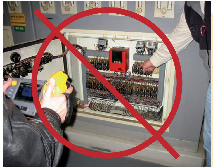
IR-Fusion eliminates the dangerous practice of sticking a finger in an electrical cabinet to show which component is overheating.
