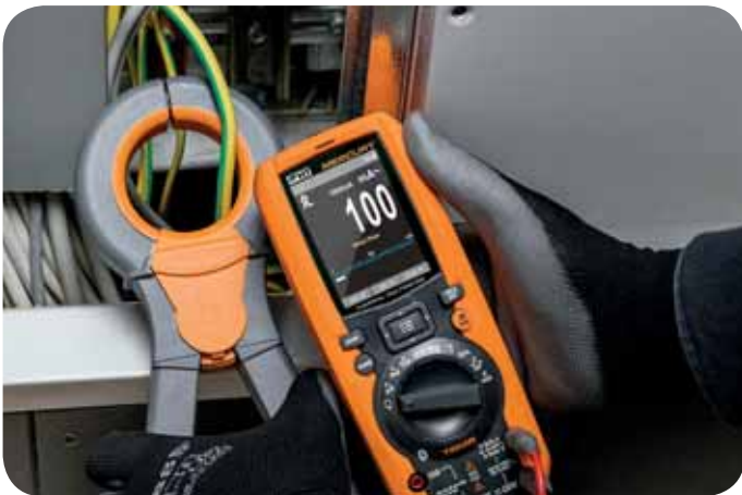
AC leakage measurement.
