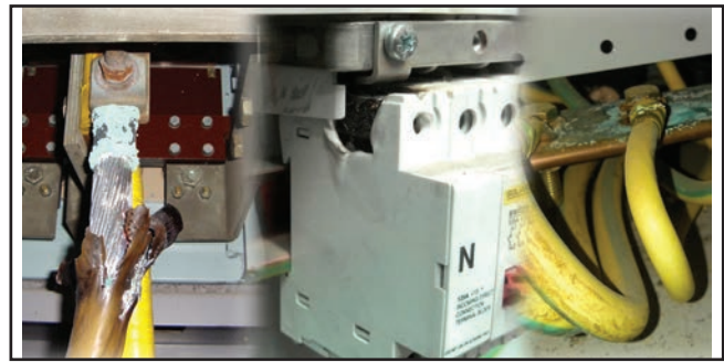
Fig 16: Typical faults that can be prevented by low resistance testing
