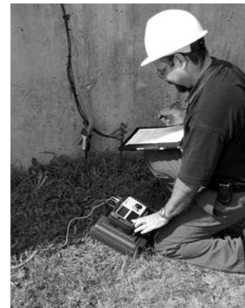
Using ART method with Megger DET3TC to test commercial ground without disconnecting the system
